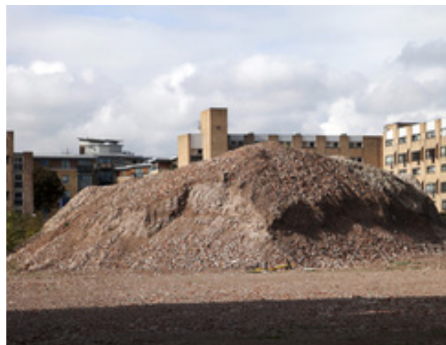
Rubble left behind in Centre of Estate
