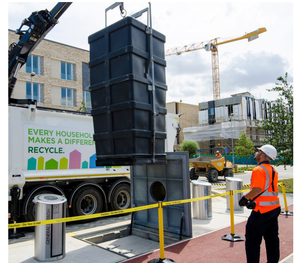
Shared Waste Service - North West Cambridge, UK
